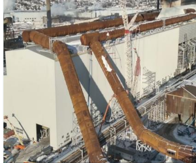
Dust system complete.
