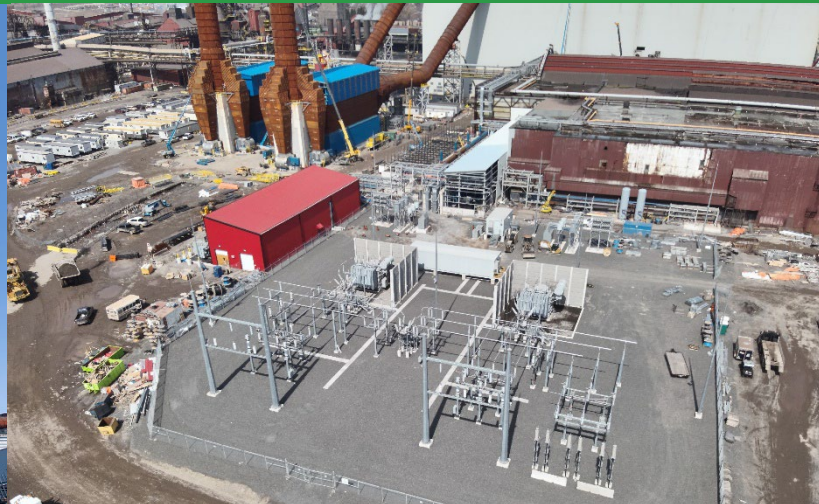
EAF Electrical Substation Tested and Energized
