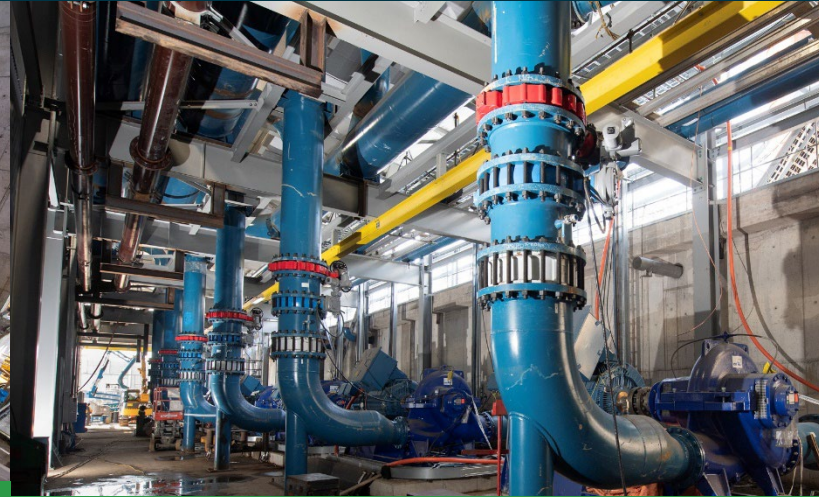
Water Treatment Plant Commissioned
