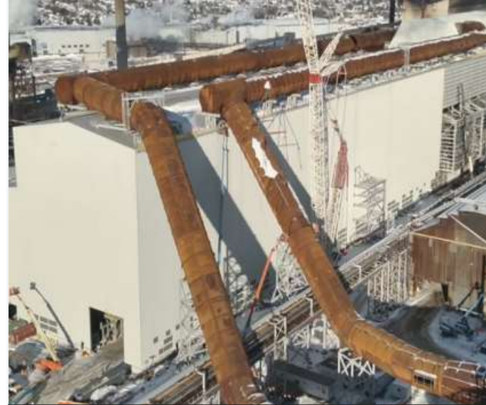
Dust system complete.
