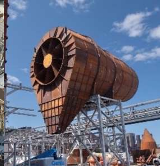
Axial Cyclone installation on Baghouse
